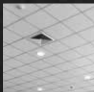
CEILING GRID FALSE CEILING
