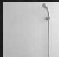
WALL CERAMIC TILES TILL 4 FEET / 7'-0" FEET HIGH & WHITE WASH/OIL BOND DISTEMPER ABOVE
